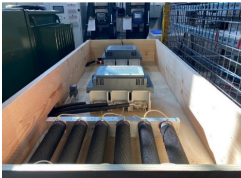
Assembly for the 480V pre-charge circuit and main contactor.
